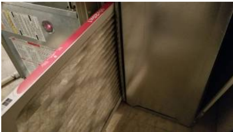
Air filter in good condition.
