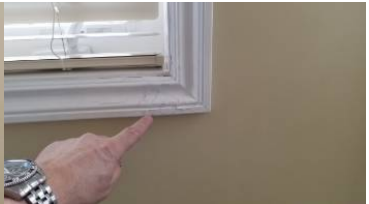
Evidence of previous leaking.
