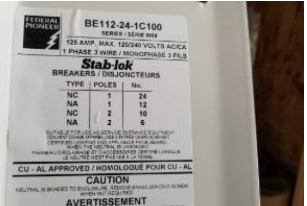
Main panel manufacturer information.
