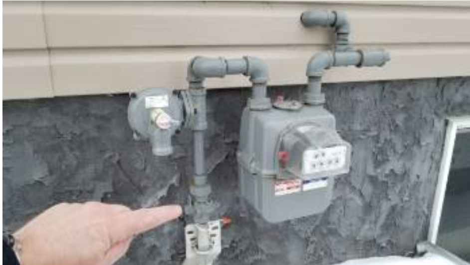
Main gas shut off valve.
