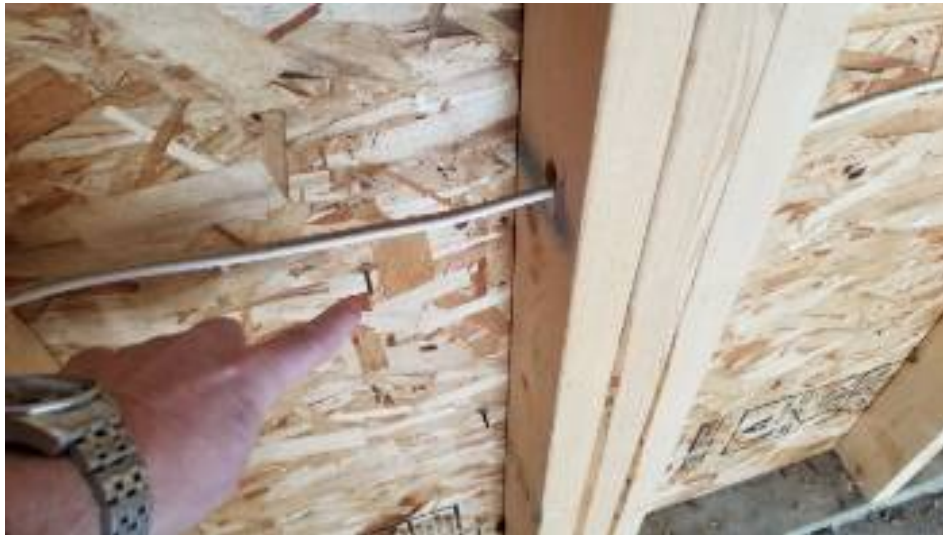
Sharp nails protruding.
