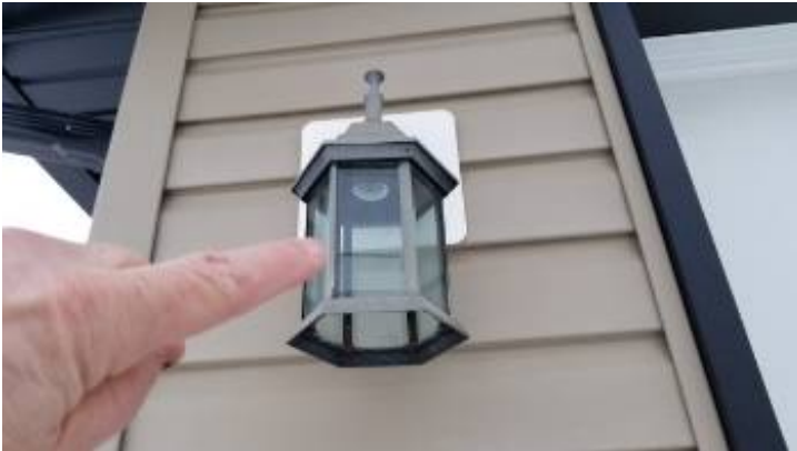
Missing light bulb.
