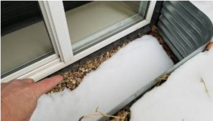
Window too close to ground.
