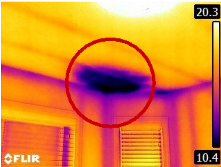
Infrared anomaly in second (front) bedroom.
