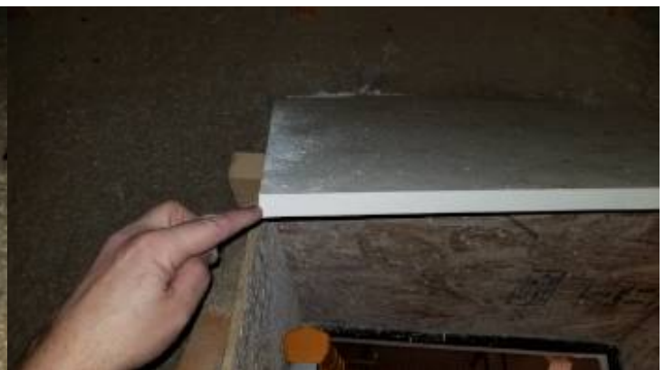
Insufficient hatch cover insulation.
