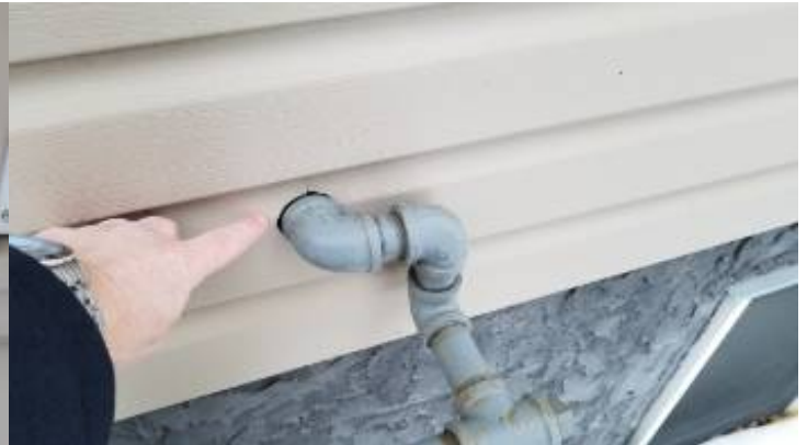
Unsealed through-wall penetration.
