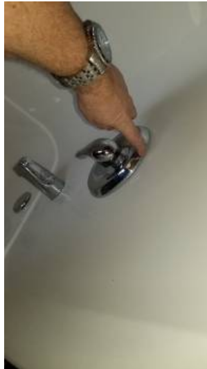
Loose/unsealed water valve escutcheon.
