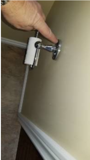
Loose toilet paper holder.
