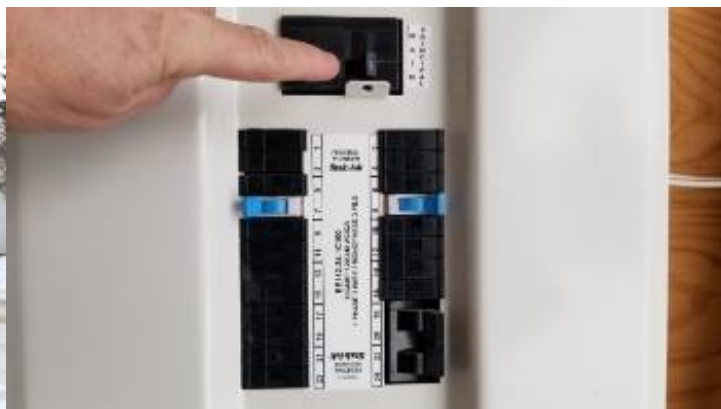
100 Amp main disconnect.
