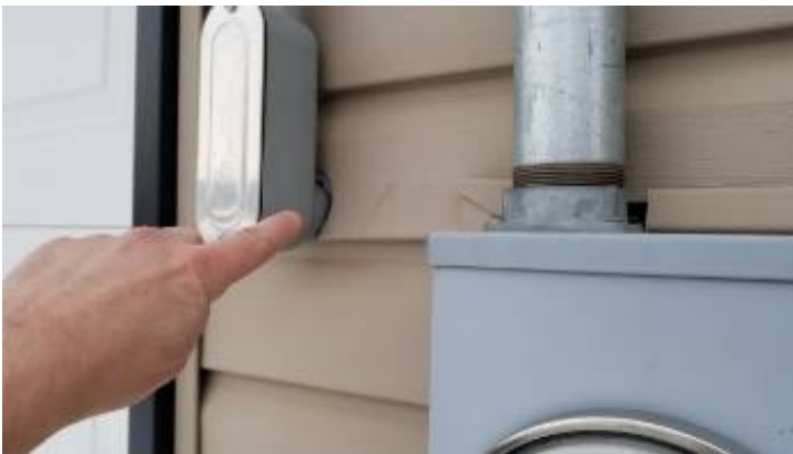
Unsealed through-wall penetration.
