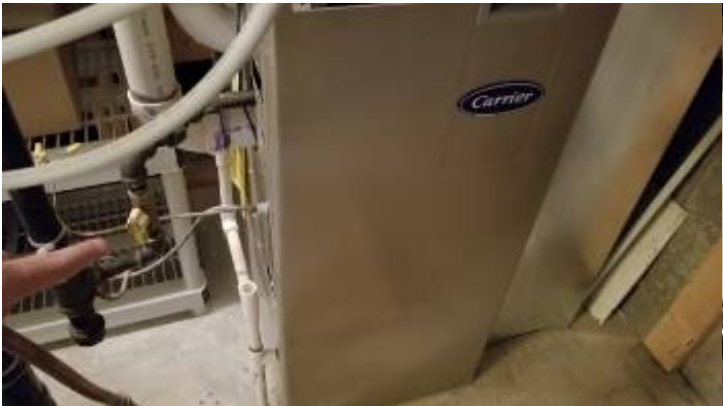
Gas shut off valve.
