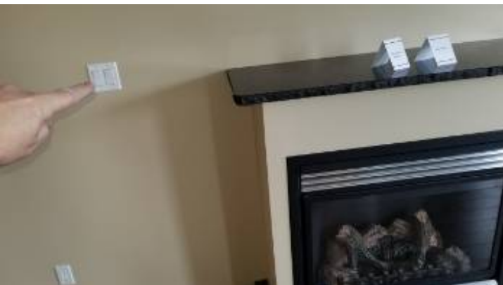
Control switch for fireplace.
