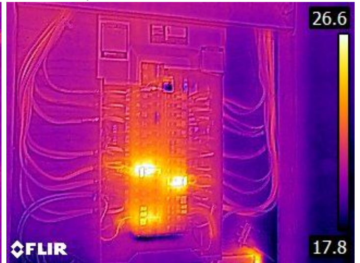
No concerns at sub panel.
