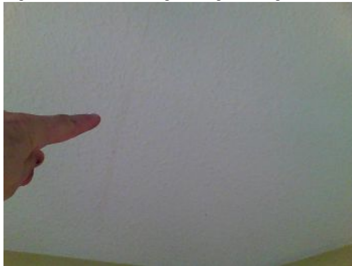
Staining at area of anomaly.
