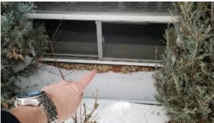
Window too close to ground.
