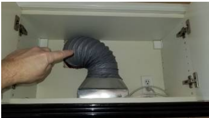
Plastic exhaust ducting.
