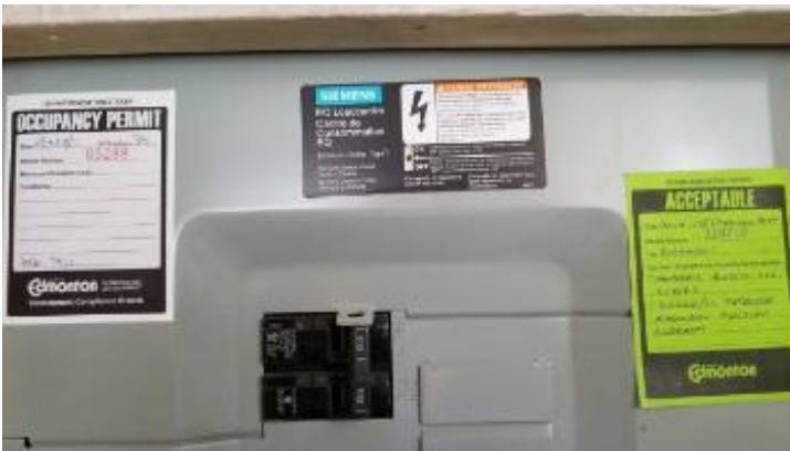
100 amp main disconnect on sub panel.
