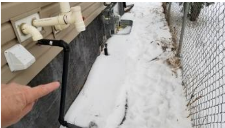
Sump discharge line.
