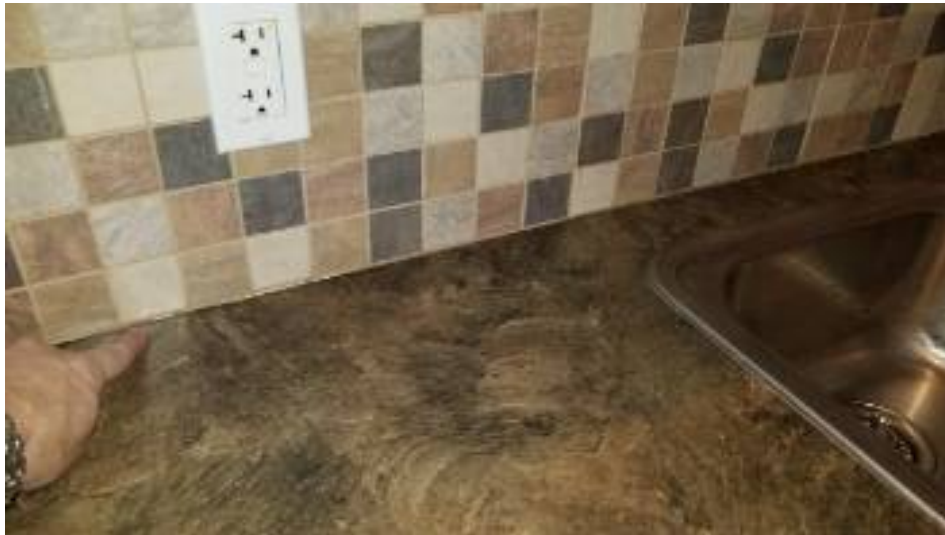
Caulk sealant required.
