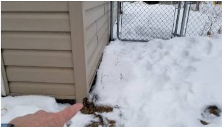
Damaged siding corner piece.
