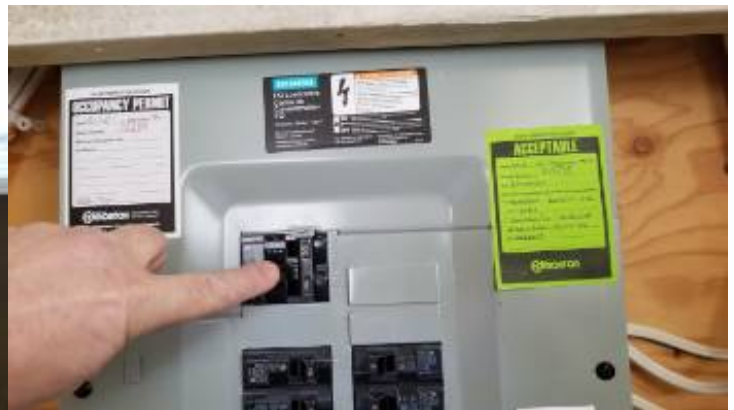
100 Amp main disconnect on sub panel.
