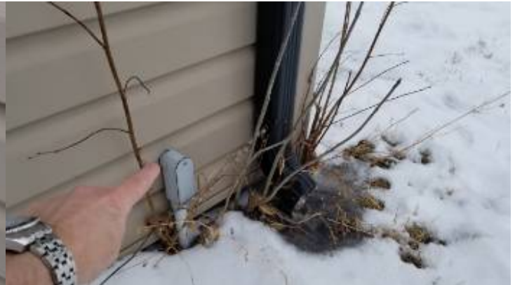
Unsealed through-wall penetration.
