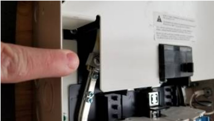
Aluminum service entrance cables.
