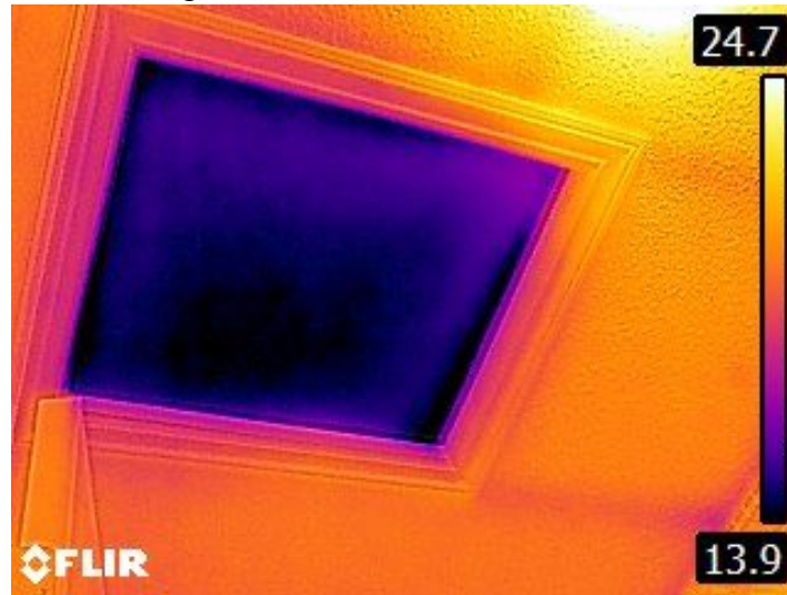
Hatch cover not insulated.
