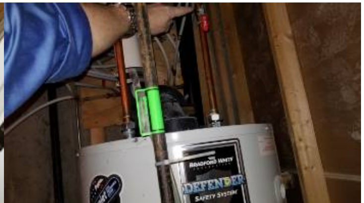
Water shut off valve.
