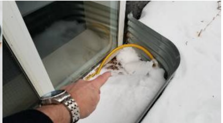
Window too close to ground.
