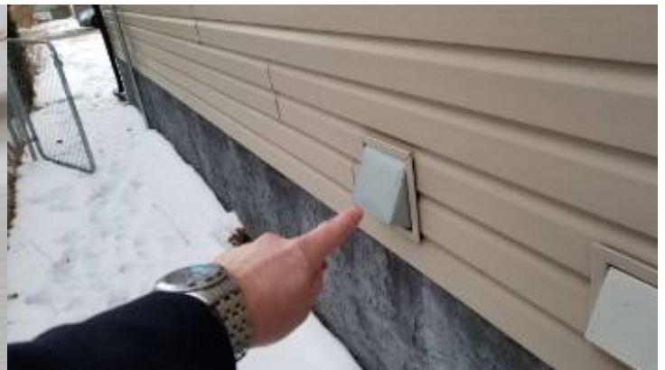
Dirty/blocked air intake screen.
