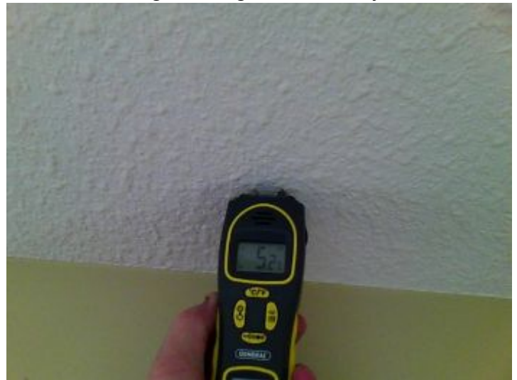
Digital image of moisture reading at anomaly.
