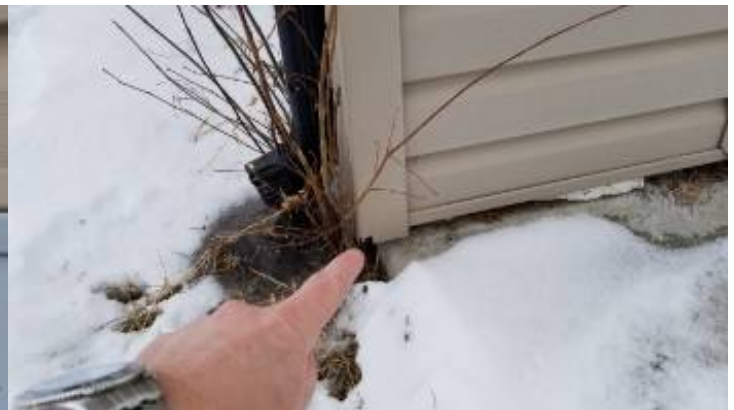
Damaged siding corner piece.
