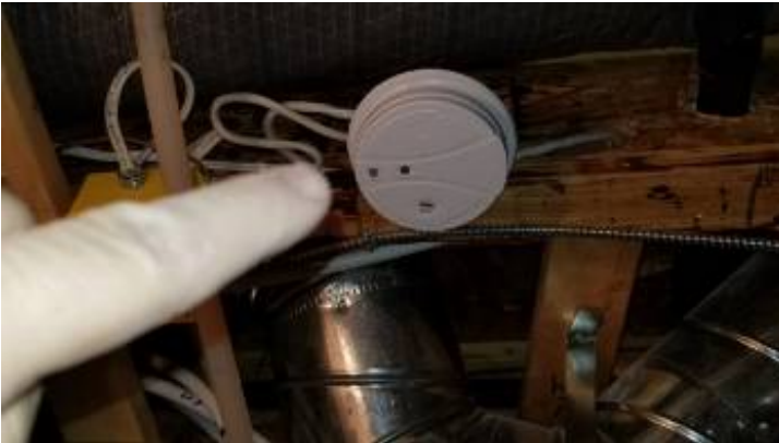
Basement furnace room.
