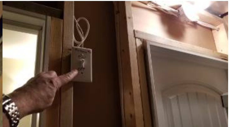
Electrical shut off switch.
