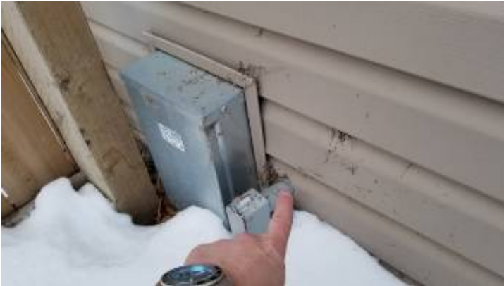
Unsealed through-wall penetration.
