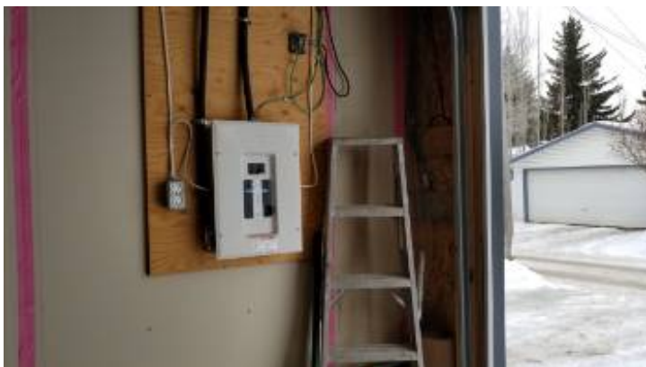
Main panel located in garage.
