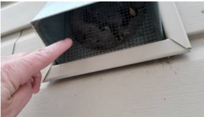
Dirty/blocked air intake screen.
