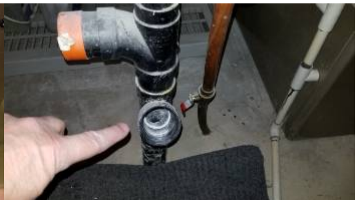
Open clean out/waste line.
