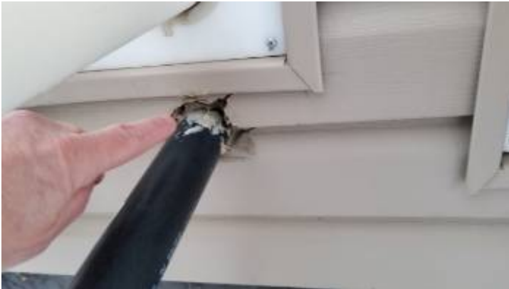
Unsealed through-wall penetration.
