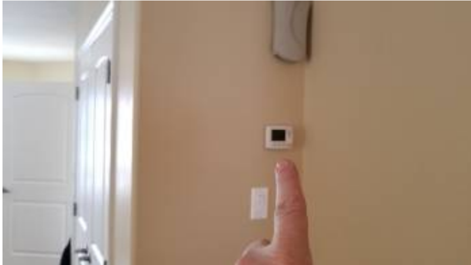
Heating unit thermostat.
