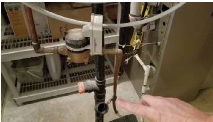
Main water shut off valve.
