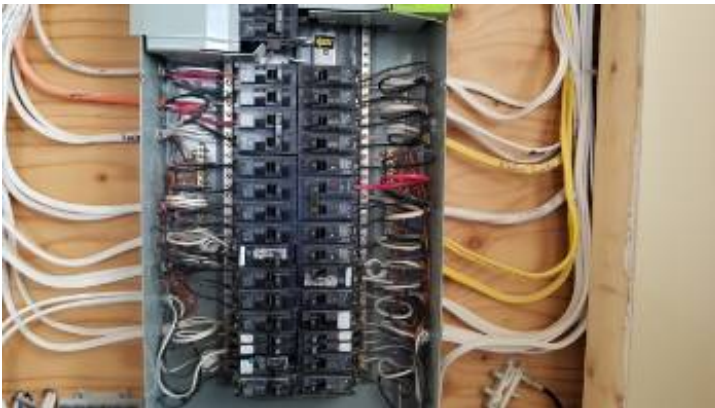
No concerns noted in sub panel.
