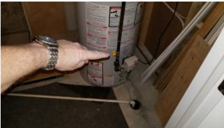
Gas shut off valve.
