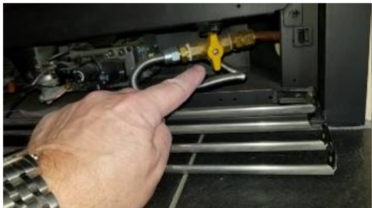
Gas shut off valve for fireplace.
