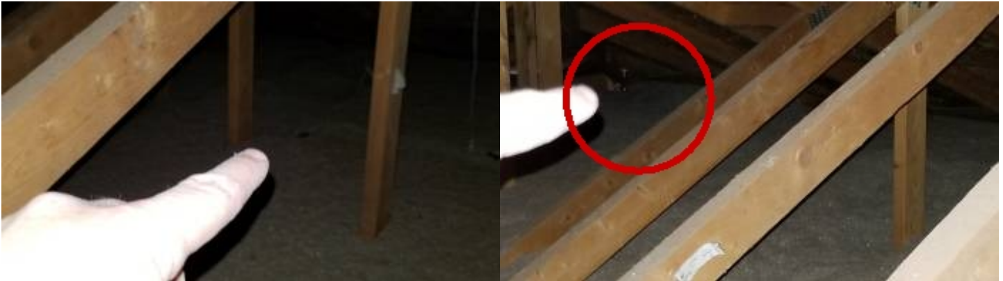
Uneven insulation coverage.
